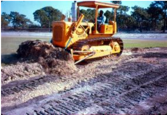
Birch used all available resources to complete field renovation projects. Here, a grader and skilled operator, borrowed from another department, work on a field.
